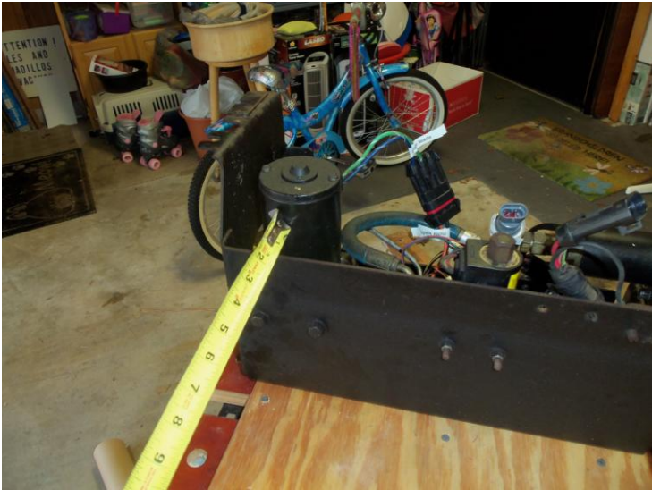
The hydraulic pump, which will be removed.
