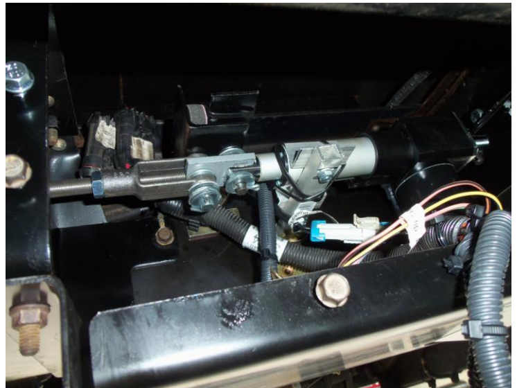
The installed park brake unit with the actuator retracted (brake on).
